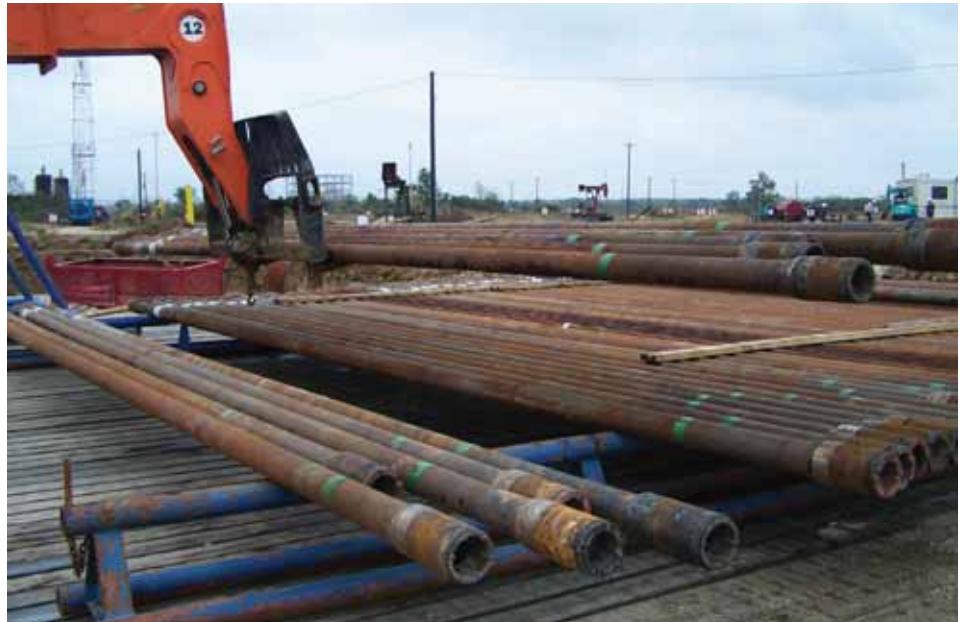
The pipe pictured above will be used to drill a well deep into the Spindletop salt dome. The process takes several months. Once complete, the well will then be used in the leaching process, in which water hollows out the storage caverns.
