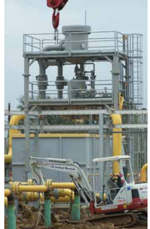
The water-handling facilities manage the flow of fresh water into the cavern well and pull the salty water, or brine, back out. The equipment pictured above is a hydrocyclone filter. It removes insoluble materials from the brine after it is removed from the cavern and before it is pumped to the brine disposal wells.
