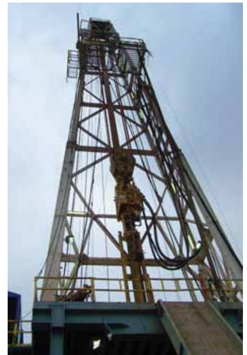
Crews set up the rig on the second cavern site and drilling began in early December.
